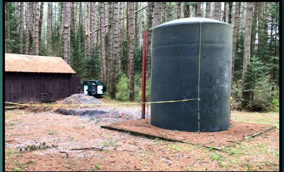
Water Storage Tank
